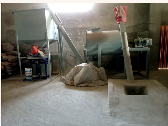
Blending equipment in the Rawat facility.
